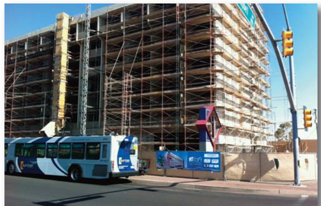
aloft hotels, a Starwood brand, is conducting several conversion projects this year in order to quickly expand the aloft experience to new markets. Pictured above is the construction site of aloft Tucson, Arizona, a former Four Points by Sheraton Hotel. JN+A and HVS Design are providing Architecture and Interior Design Services for the project.
